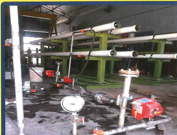
RO SYSTEM SS 316 L & MEMBRANE AUTO SYSTEM
